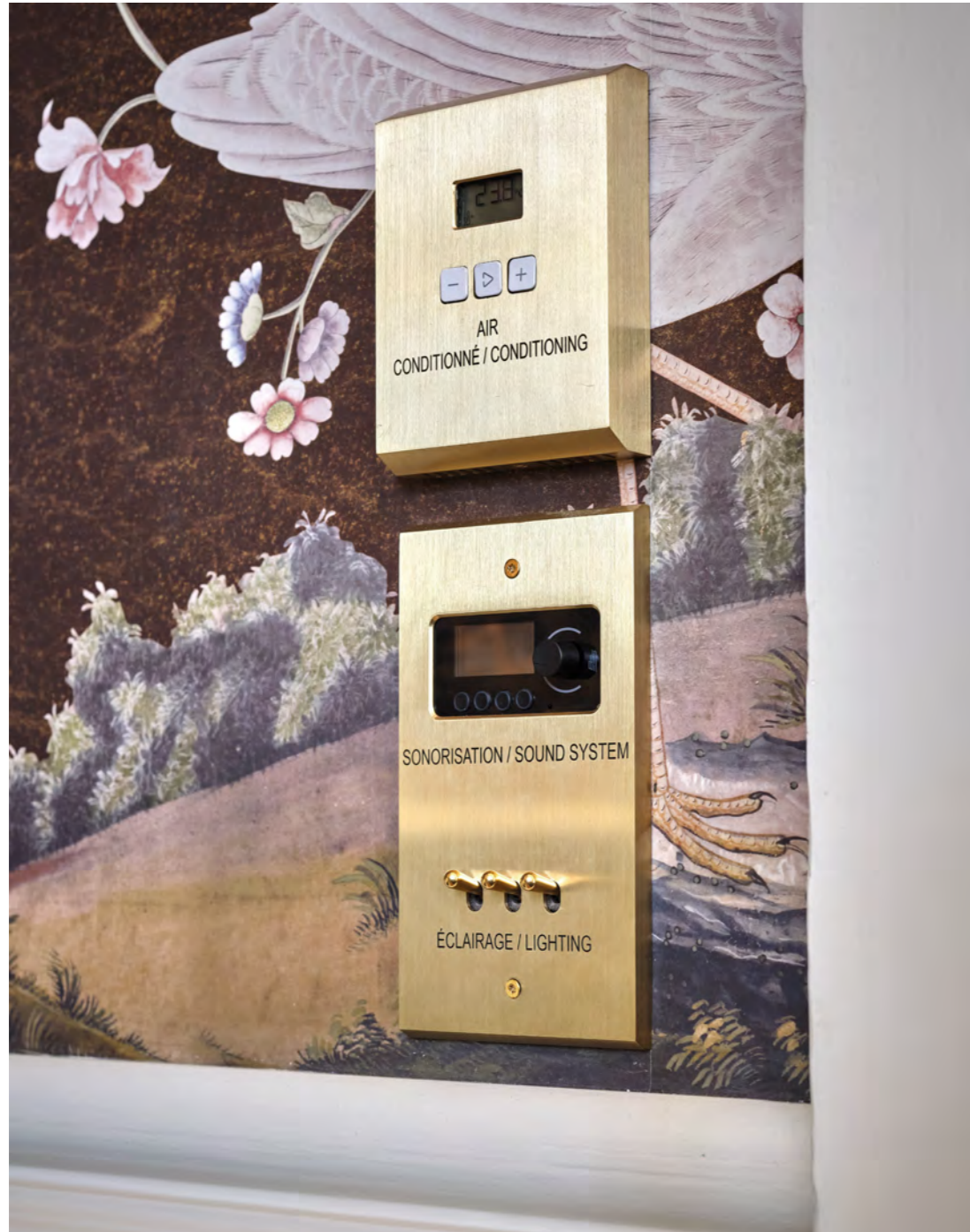
Above, Confidence collection, custom brushed brass plate for air conditioning and sound system, gilt toggles
